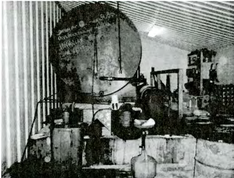
Picture 14 : Waste oil reservoir, Inukjuaq (water and antifreeze drain at bottom)
